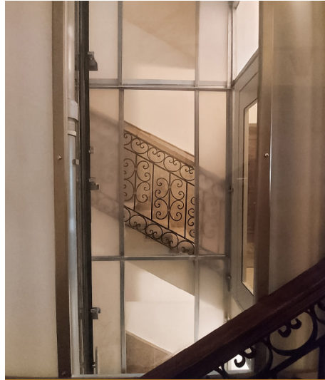
Acrylic Sheets Housing for Elevators
