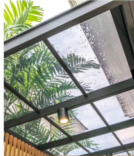
Acrylic Sheets Covers for Skylights
